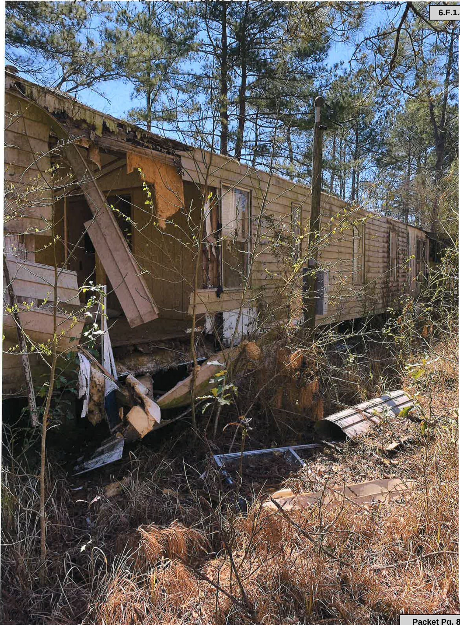
Attachment: 16070 Old Joe Moran Rd. (8030 : Safety Hazard Properties.)
